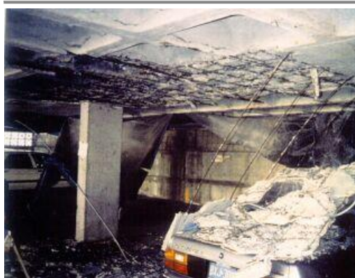
The result of spalling and rebar corrosion in garages. The proper use of deicers can help prevent this problem.
